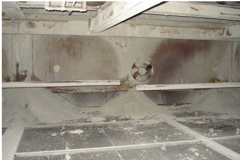
Figure 14. Reactor 3A Top Catalyst Layer Condition, May 24, 2010
