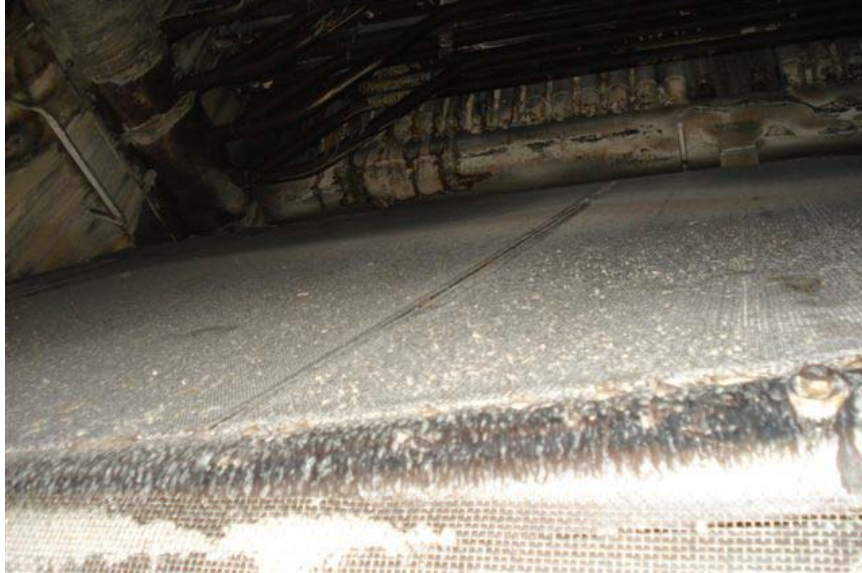
Figure 13. Upper LPA Screen Condition, May 24, 2010
