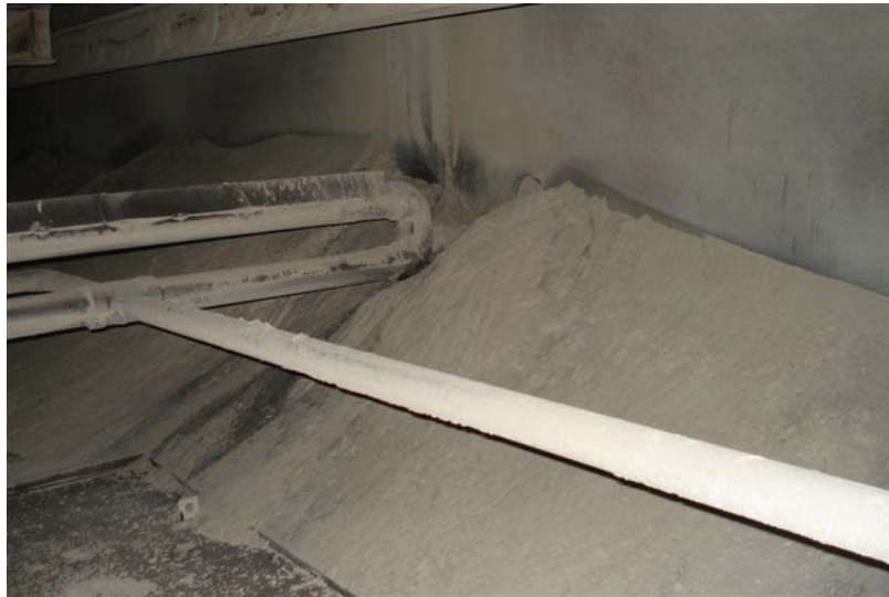
Figure 15. Reactor 3B Top Catalyst Layer Condition, May 24, 2010
