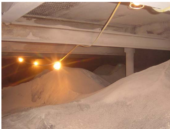
Figure 6. Typical Ash Accumulation on Catalyst Layers Before Vacuuming
