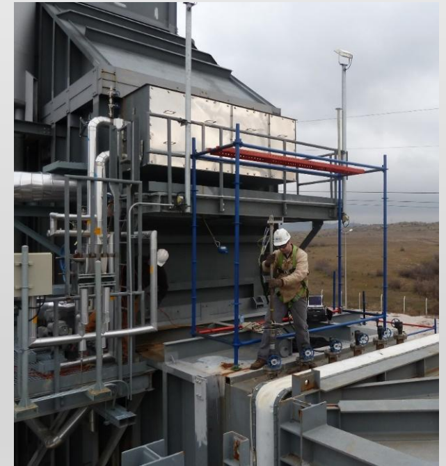
GT outlet flow measurement
